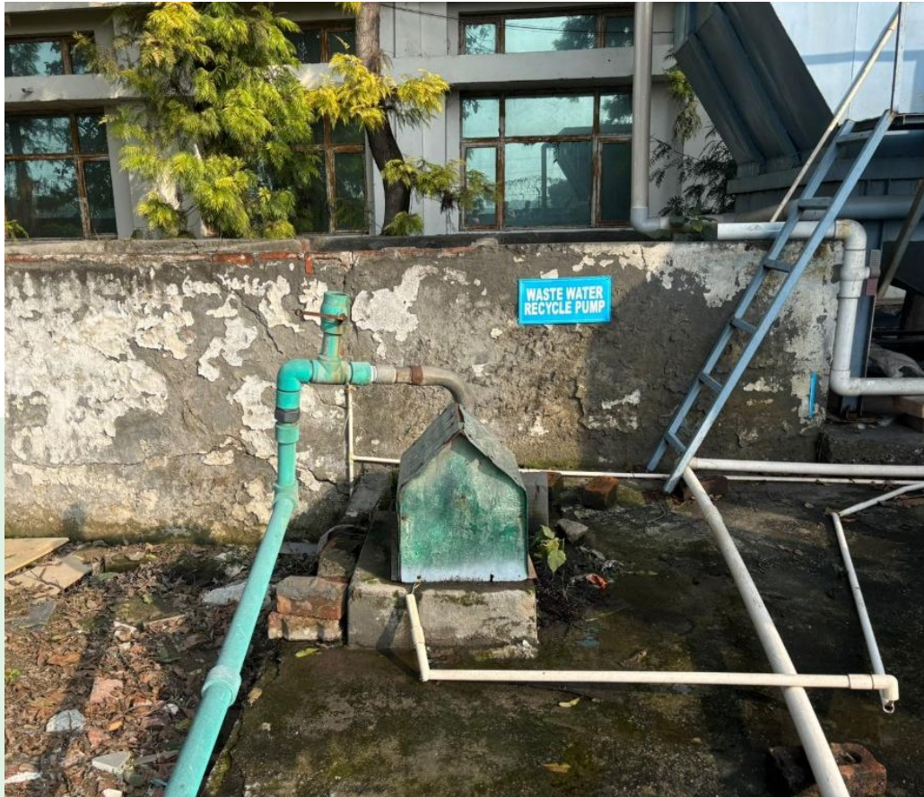
Wastewater Recycled Pump used to recycle the wastewater for the entire campus
