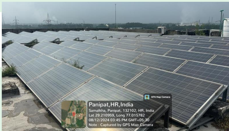
An array of solar panels installed on the rooftop of a D-Block building in PIET
