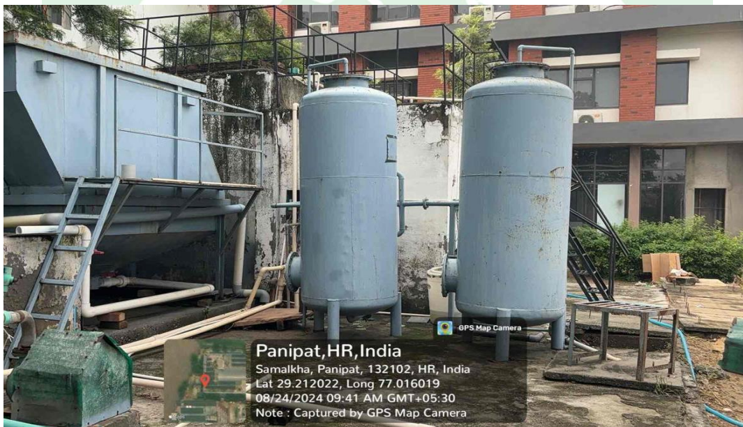
Side view of sewage treatment plant
