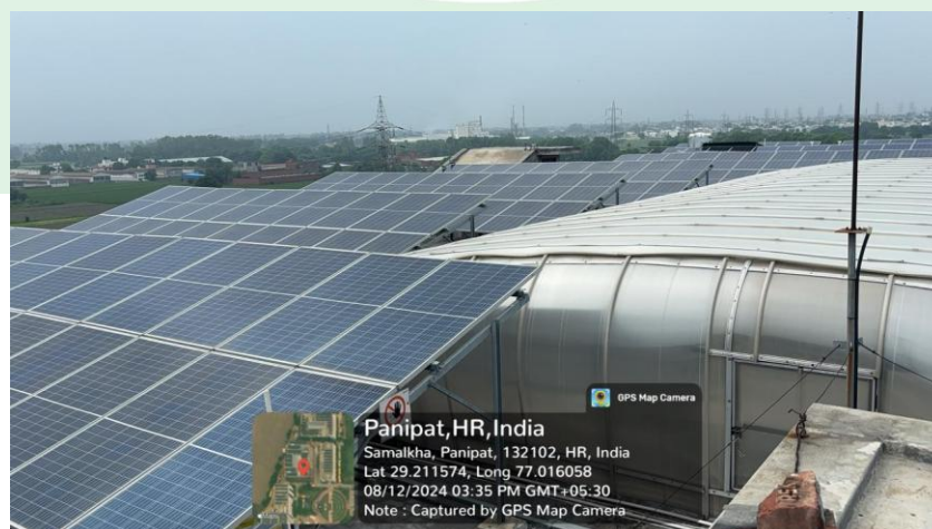
An array of solar panels installed on the rooftop of a G-Block building in PIET
