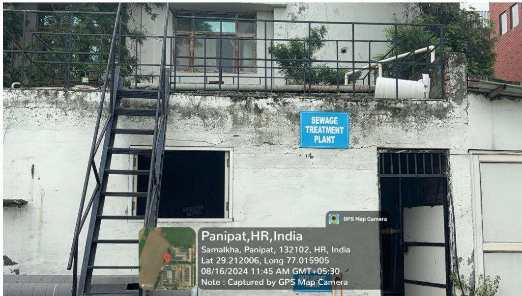
Sewage treatment plant of capacity 36000 litres per day
