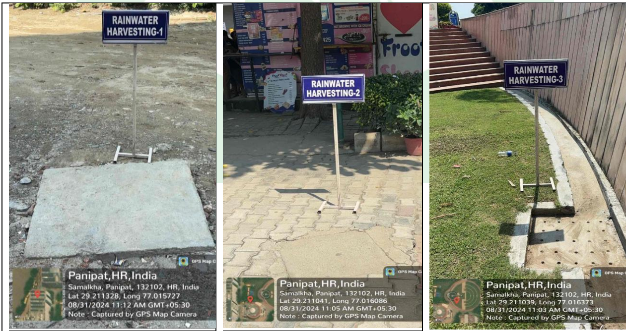
Few Rainwaters underground harvesting pits in PIET
