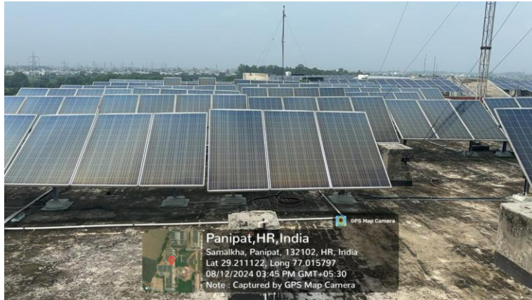
An array of solar panels installed on the rooftop of an E-Block building in PIET
