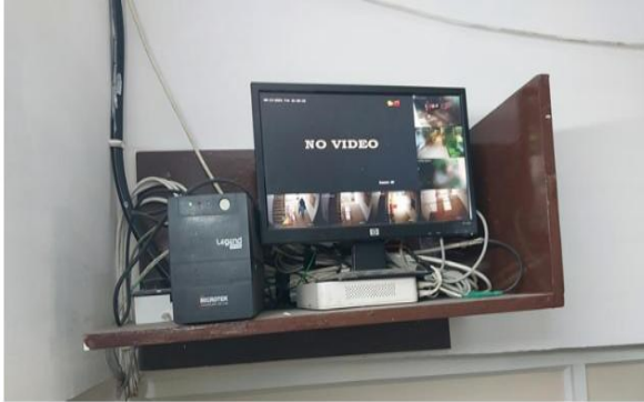
CCTV Monitoring in Himadri Girls Hostel
