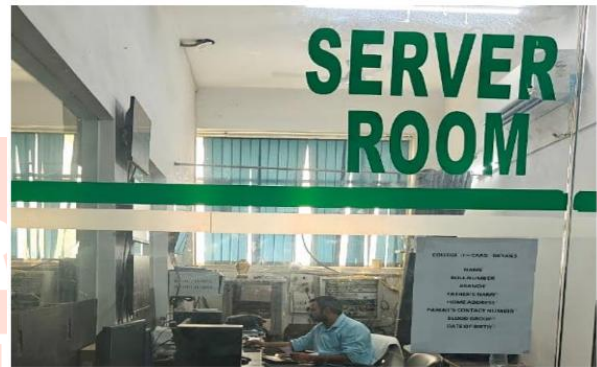
Central Monitoring Server Room
