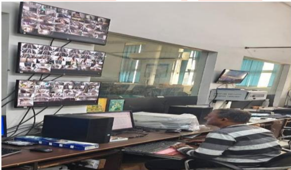
Central CCTV Monitoring Server Room
