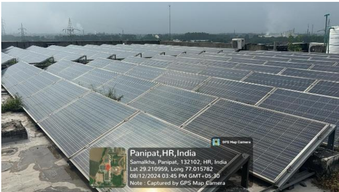
An array of solar panels installed on the rooftop of a D-Block building in PIET
