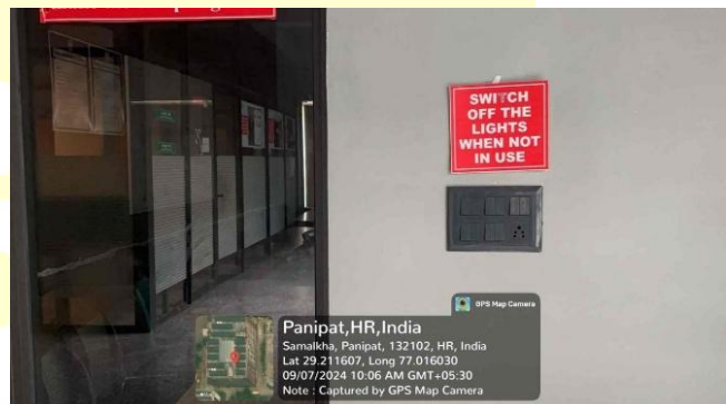
Energy conservation slogan at the main switchboard in G-Block
