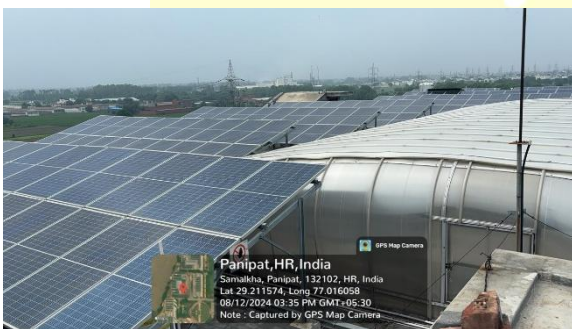
An array of solar panels installed on the rooftop of a G-Block building in PIET
