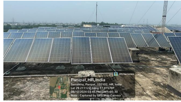
An array of solar panels installed on the rooftop of an E-Block building in PIET
