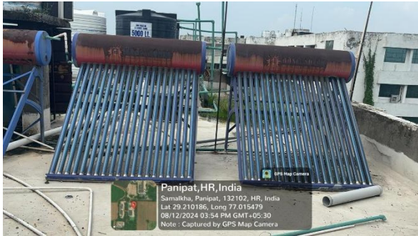
Solar Water Heater Installed on Rooftop of Boys Hostel
